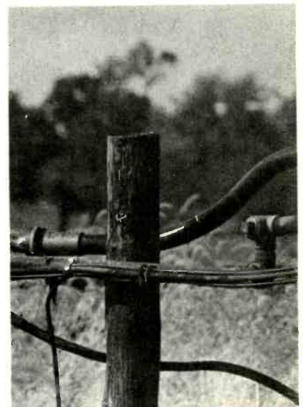
Fig. 4. Right-angle joint separated, was replaced with a curved section.
