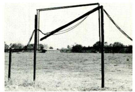
Fig. 8. Poor maintenance has allowed a wooden cable support to collapse.
