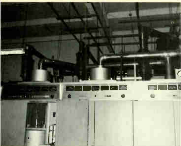
Fig. 5 View of aural and visual klystron power amplifier cabinets with attached wave guides.
