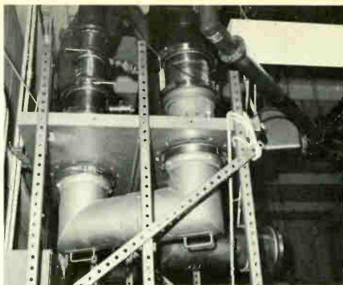
Fig. 6 Coaxial patch panel.
