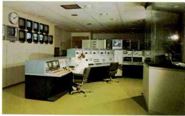
Systems-integrated Custom Audio and Video Switching . . . providing superior performance, long-term reliability at KIRO, Seattle, Washington.
