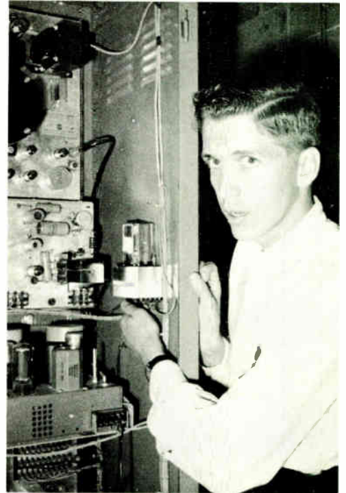
Compensator mounted inside equipment rack behind modulation monitor.
