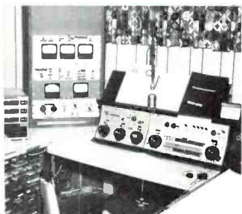
Fig. 4 AM control room with AM remote control and switching unit at center. The AM transmitter remained in the old station facility.
