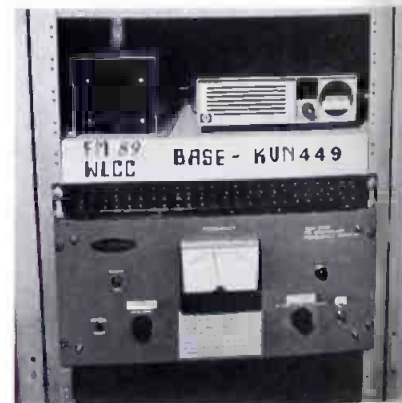
The RF 1500 transceiver and power supply are shown here in an equipment rack in WLCC's engineering room.
