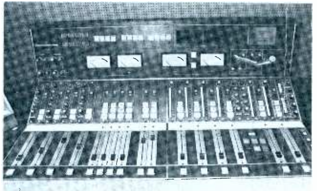
Figure 7 The WABC production control room 8C console, shown during installation, is used to make pre-recorded shows and promos.
