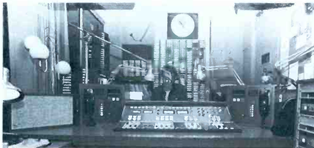
Figure 4 The WPLJ main air studio (FM-1), as seen from the engineer's side, is similar to that of 8A, but faders 8-10 are used for turntables.
