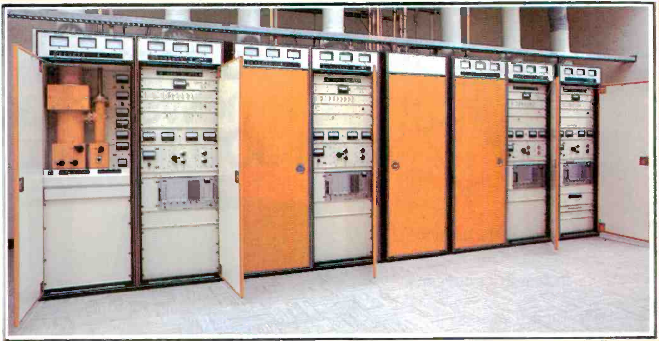
CGE Model "F" VHF TV transmitter installation at Canadian Broadcasting Corporation (CBC) station in Fort McMurray, Alberta, includes two main/alternate configurations (4 transmitters) for both English and French transmissions.
