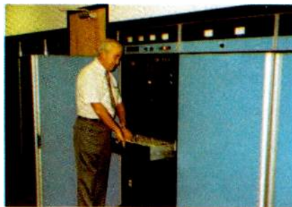
Harris 50kW transmitters at WKRC.
