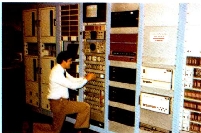
Video routing and pulse distributing at WKRC.
