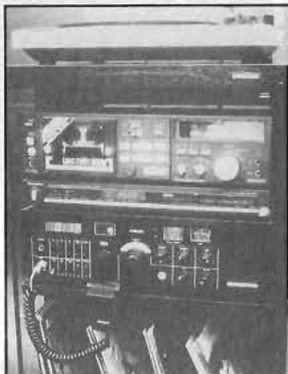
Rack system supplied by Mr Cad, Whitgift Centre, Croydon.
