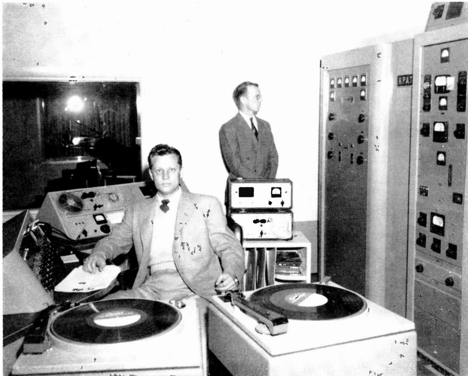
Complete GY-48 Radio Station with Gates Speech Equipment at Radio State KPAT, Pampa, Texas. Note massive appearance and excellent combination type installation.
