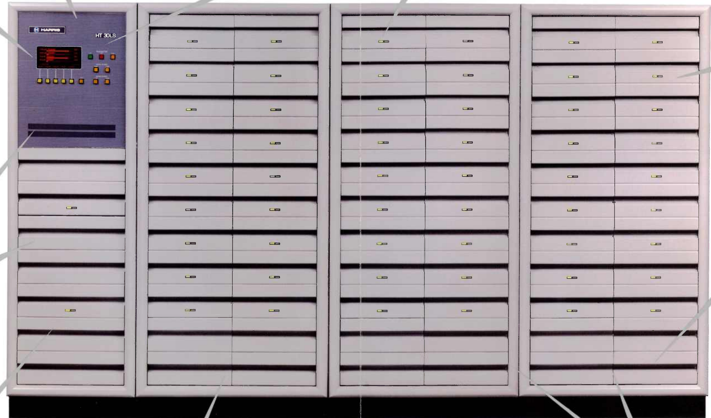
The model shown is the HT 30LS, 30 kilowatt low band solid state VHF transmitter configured with dual exciters and the 20 percent aural option.
