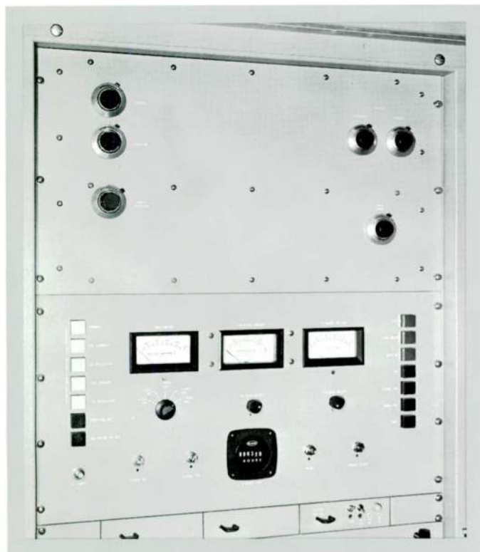
RF Monitoring, Metering and Status Light System
