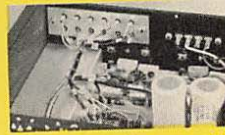
Labeled wiring harness makes point-to-point connections easy.
