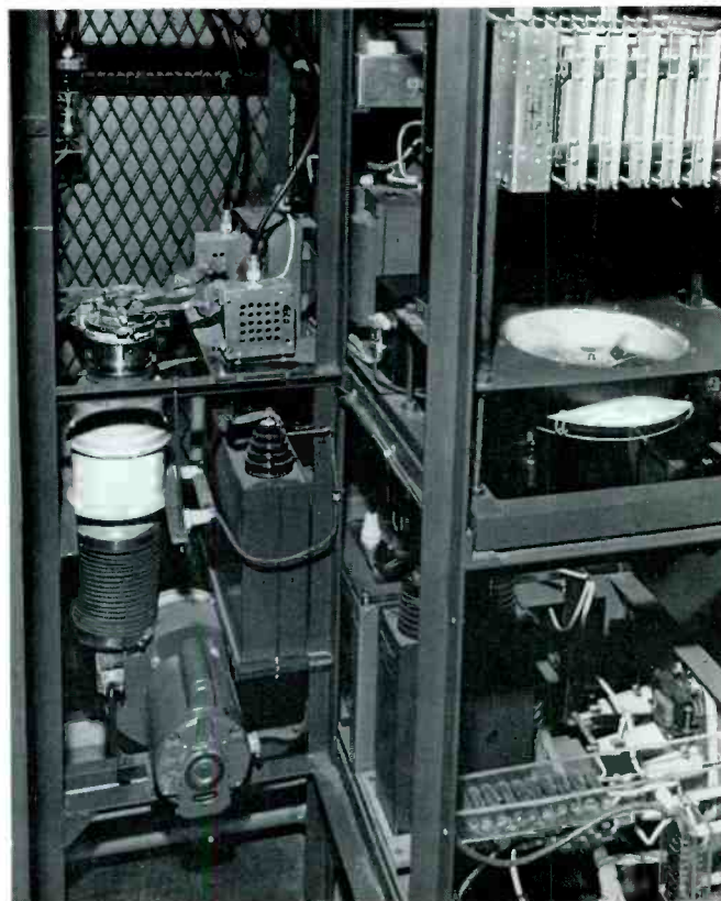
Figure 4 — Driver cubicle with access panel removed.
