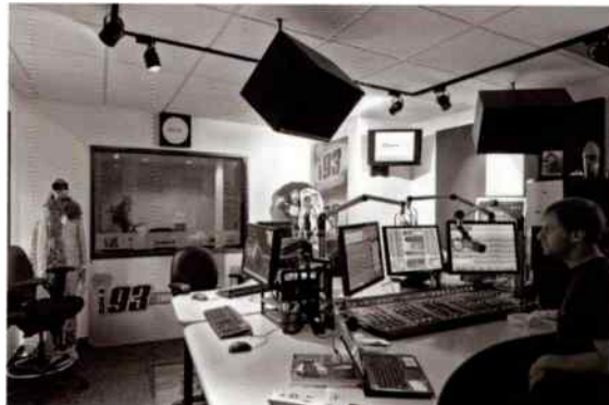
Talent at the Axia Element console in 193's air studio. Note the Telos Call Controller built into the console, which directly controls the Telos VX Broadcast VoIP phone system.
