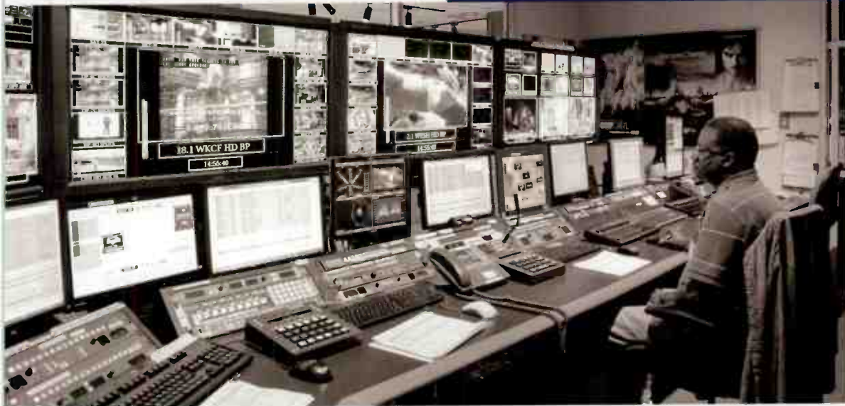
MASTER CONTROL OPERATIONS AT HEARST AFFILIATE WESH IN ORLANDO, FLORIDA
