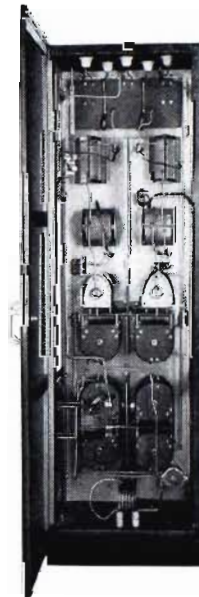
Interior view of a 1 KW phasing and branching equipment
