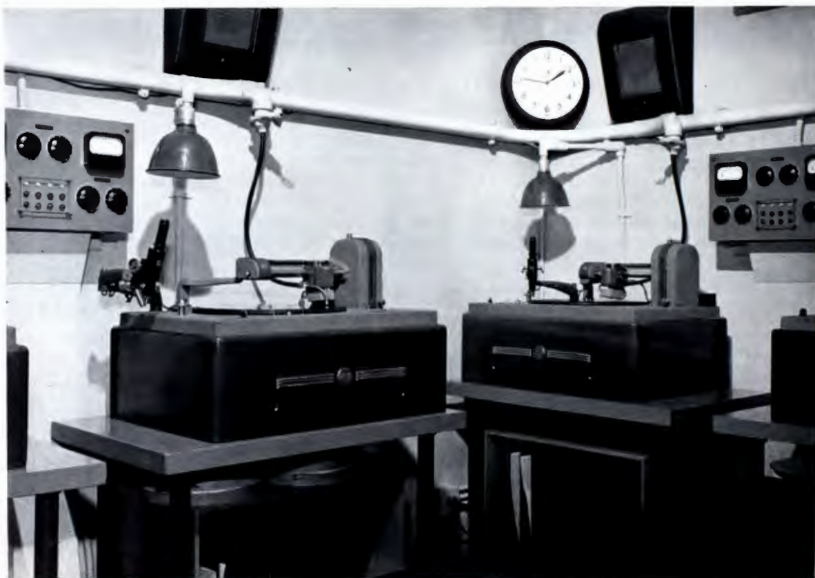
◀ An ideal recording installation at KECA, Los Angeles, Calif., showing two of the four RCA 73-B Professional Recorders. Note the conveniently located overhead lighting, the large size auction duct, and relatively short length of hose for chip removal.
