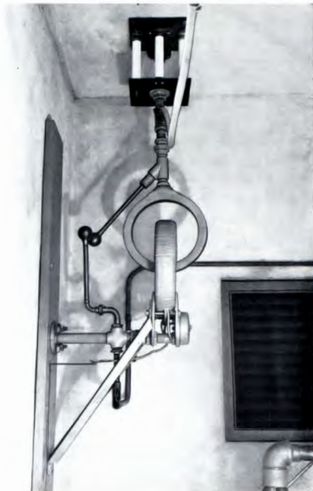
Typical Installation of an Austin Tower Lighting Transformer
