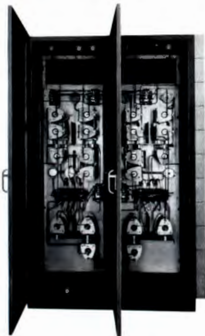
Open-door view of the equipment in an MI-28935-B Cabinet
