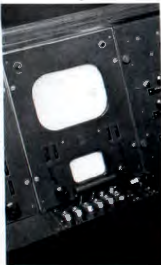
Closeup of TS-10A Control Panel
