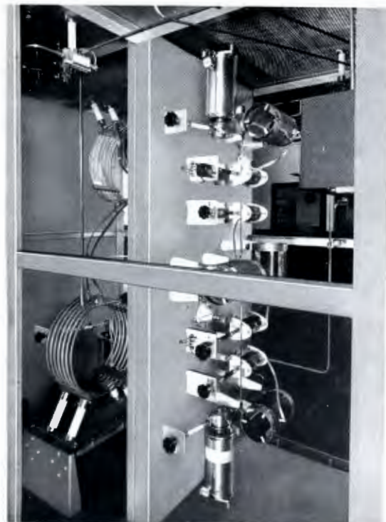
Interior view of a 50 KW phasing and branching equipment
