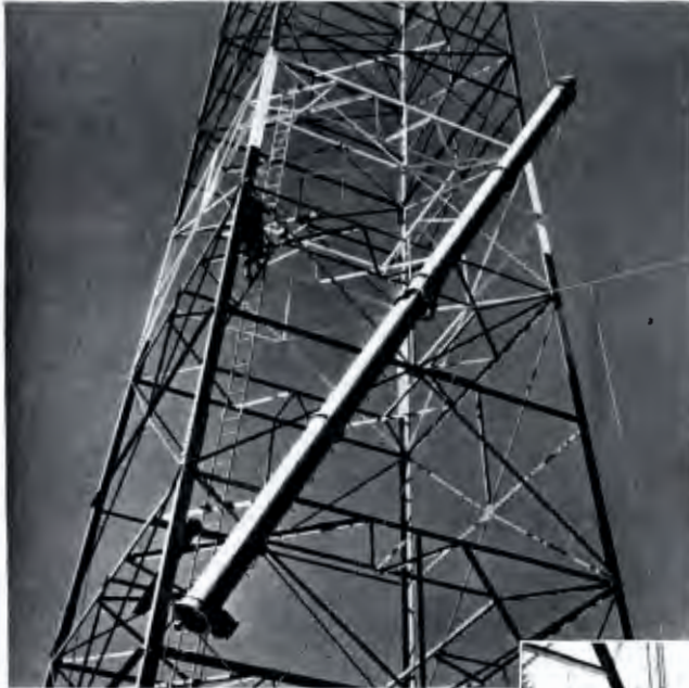
Raising the four-section Pylon in one completely assembled unit at WJPG-FM, Green Bay, Wisc.
