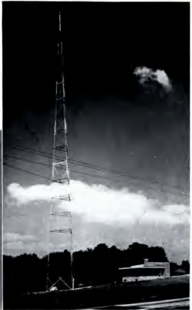
Tower and two-section Pylon at WSBA-FM, York, Pa.
