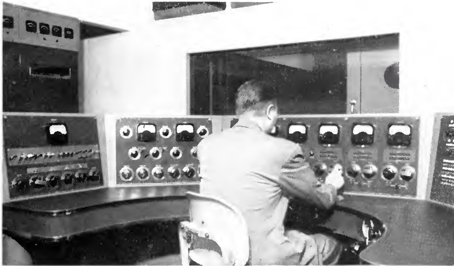
KOMO, Seattle. This master control console—with 9 deluxe audio equipment racks (at rear, not visible)—is one unit of KOMO's completely new and modern 7-studio system. It incorporates complete center panel switching for 10 studios and 6 outgoing channels (KOMO-AM, KOMO-FM, network plus 3 emergency).
