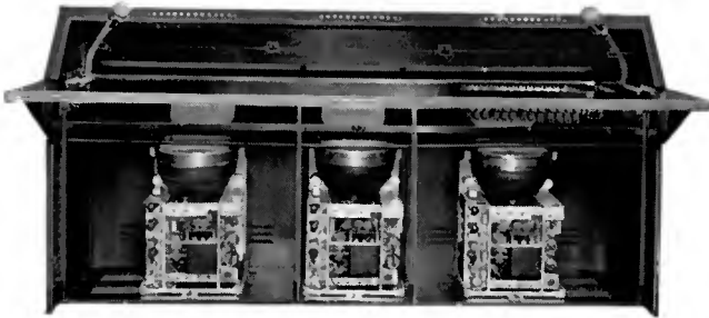
TC-5A front cover removed to show mounting of monitors
