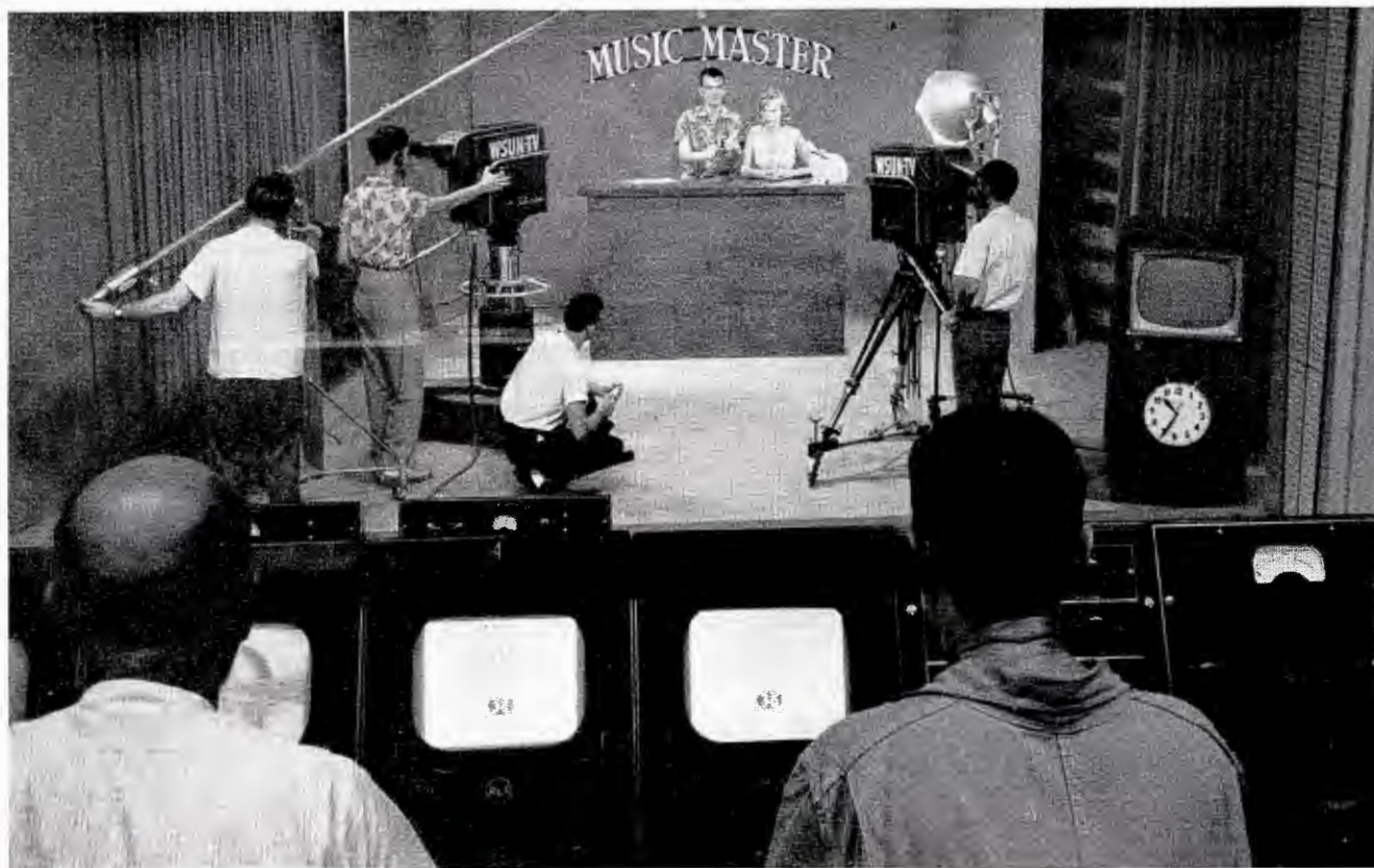
Two complete RCA Studio Camera Chains are shown installed in the studios of WSUN-TV, St. Petersburg, Florida.
