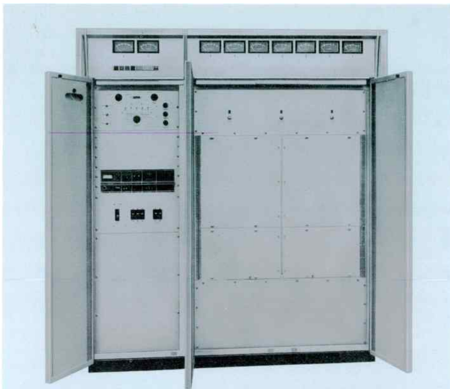
Front view, doors open. Note exciter unit.
