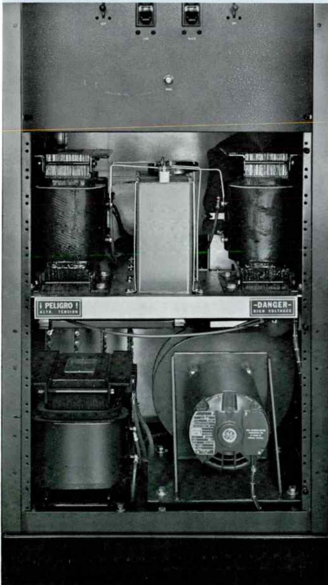
Lower front with access panel removed showing oversize blower, plate transformers and reactors.
