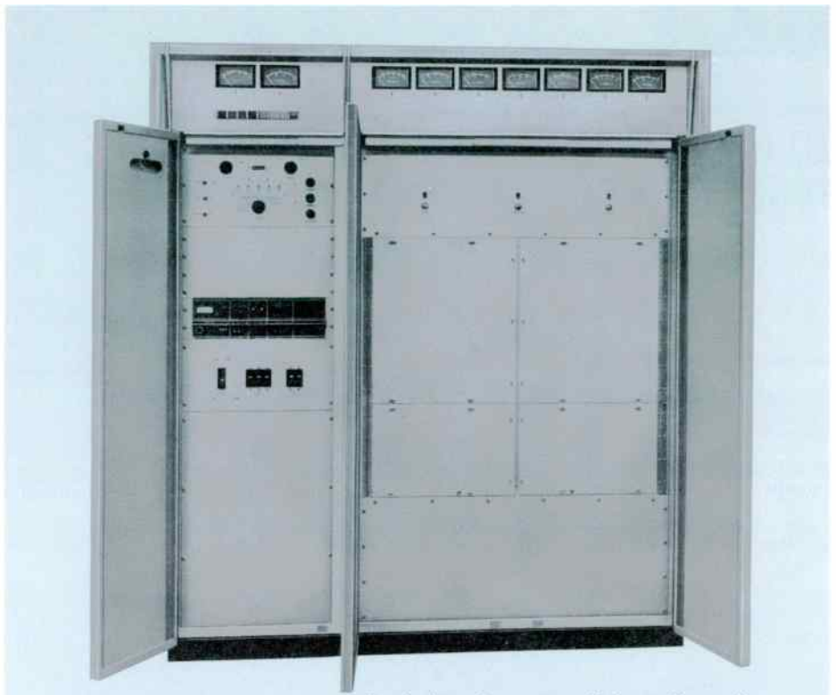
Front view, doors open. Note exciter unit.
