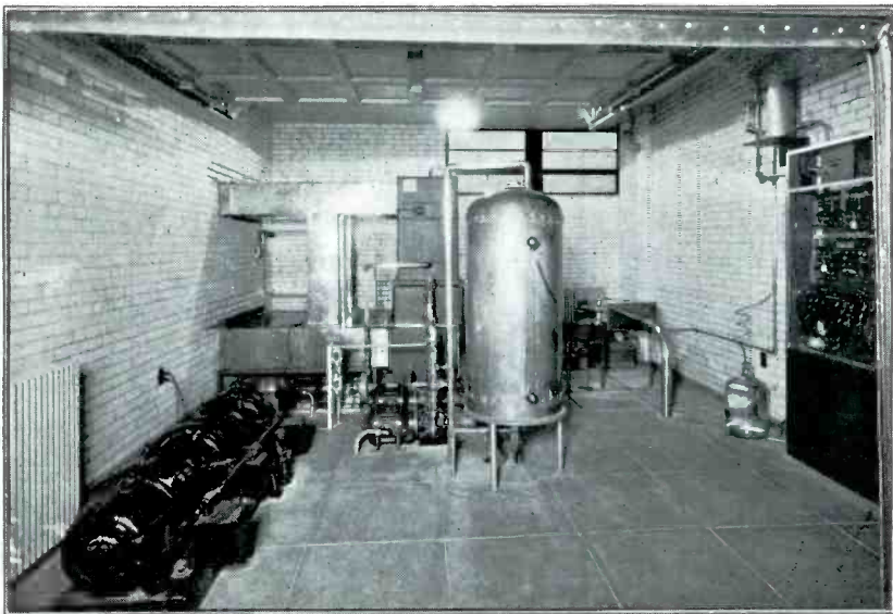
FIG. 9. THIS ARRANGEMENT AT PAXTON, MASS. IS SIMILAR TO W55M LAYOUT, SHOWN IN FIG. 7
