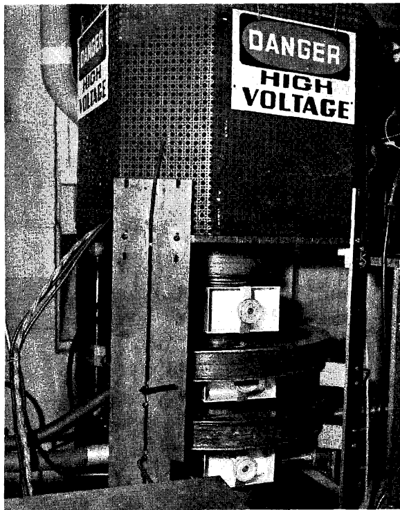
Fig. 8—The 5-kw klystron on test.
