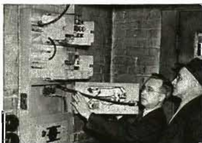
William G. Clinton, DT&I communications engineer, showing induction unit to Emery Lee, FCC inspector.
