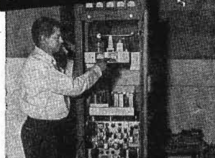
Typical Motorola transmitting and receiving unit as installed for Miami Police Department.
