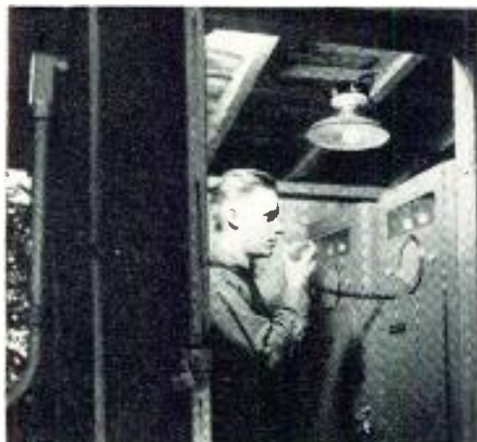
Taking a meter reading at the central station installation on Selden Hill.
