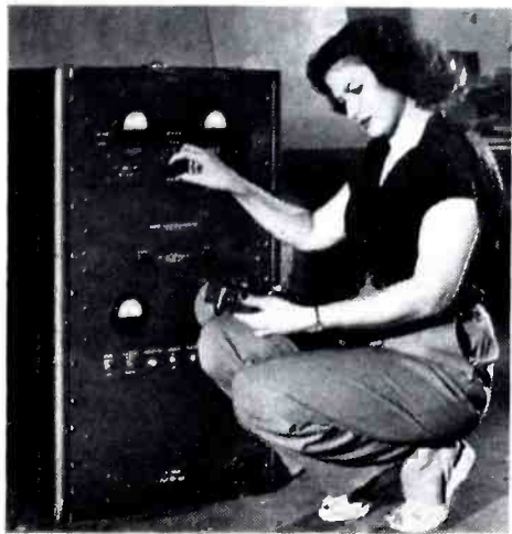
Mobile Communications control cabinet used in the Yellow Cab System.
