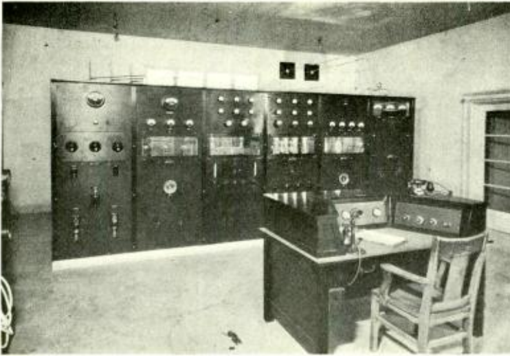
View of the transmitter room at KOL, Seattle, Washington. The transmitter is a 5000-watt job, crystal controlled, 100-per cent modulated. Air-cooled rectifier tubes are employed.
