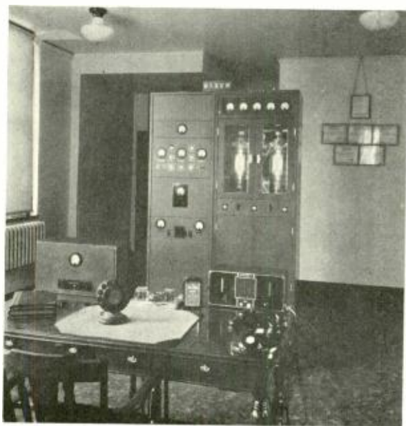
The panel at the left is the 50-watt ultra-high-frequency transmitter. The one at the right is the 500-watt amplifier. On the left corner of the dispatcher's desk in the foreground is the control unit and on the right corner a station-house receiver used for monitoring.
