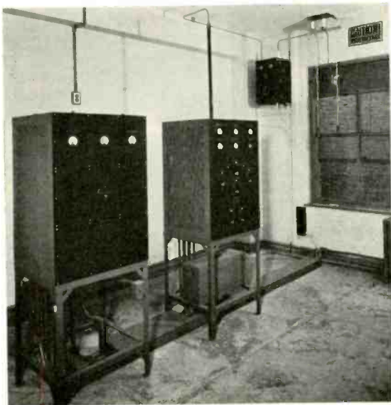
THE TRANSMITTING EQUIPMENT AT ST. GEORGE, STATEN ISLAND. OPERATION IS BY REMOTE CONTROL FROM THE RECEIVING STATION AT ROSEBANK, S. I.
