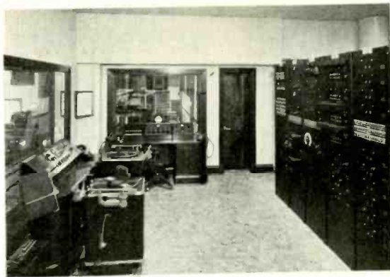
STUDIO CONTROL ROOM OF RADIO STATION WKY, OKLAHOMA CITY, OKLAHOMA.
