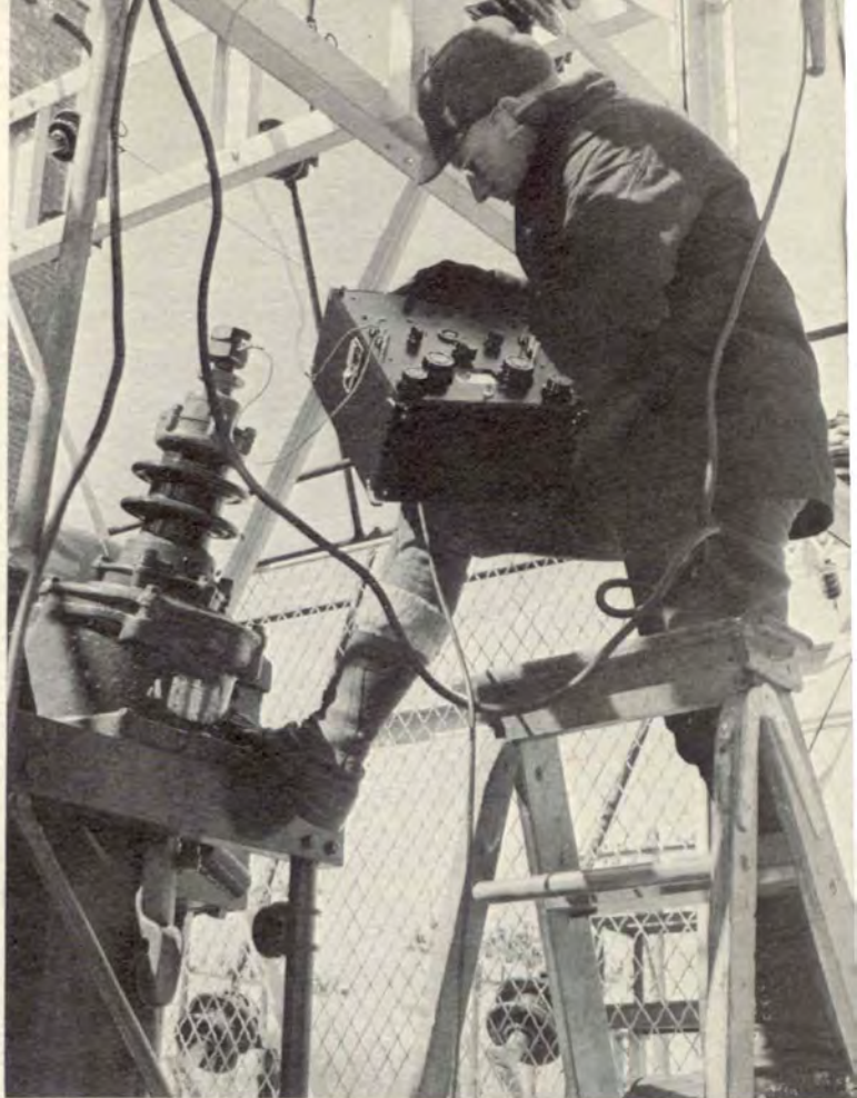
Measuring Leakage Resistance of a large power transformer with a GR Impedance Bridge. Many General Radio instruments are portable and completely self-contained, bringing laboratory accuracy to the field.
