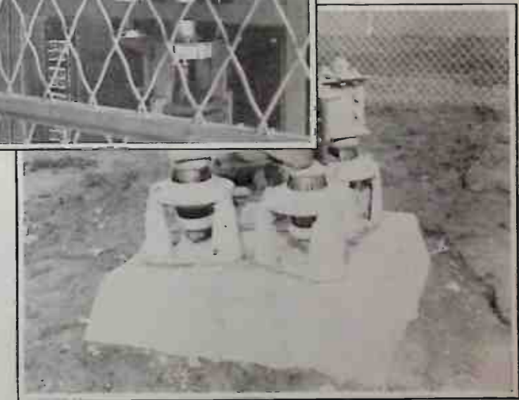
STANDING ON ITS OWN COSTLY FEET—Each tower of the WLW antenna is completely insulated from the ground. The amount of money invested in these insulators would make a sensational story.
