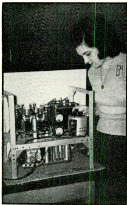
High-voltage bridge rectifier capable of delivering 0.25 amp at 2500 v with eight type 80 tubes. The Variac being adjusted here is connected across the primary of the plate transformer.
