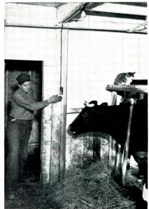
Wiring a barn, or any surface job, has been greatly simplified by Monowatt's "Surf-A-Line" plastics wiring devices. Tests were run under closely simulated farm conditions. Dust and moisture, which are ever-present in barns, were built up between two "hot" points and a normal 115 volts run through. Arcing occurred, lasted momentarily and stopped. Because the bases of these devices are made from urea compound, heat generated by the arcing dried out foreign matter and left no permanent track. After several days of this forced testing, the urea insulation still showed no signs of tracking and the device continued to operate perfectly.
