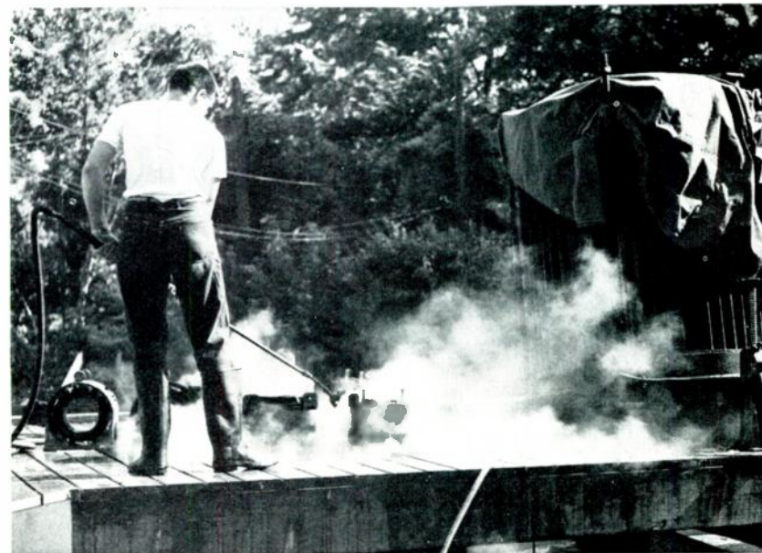
Preliminary steam cleaning of a 500-kva transformer was done thoroughly and without delay during the peak of the flood in Kansas City last summer.
