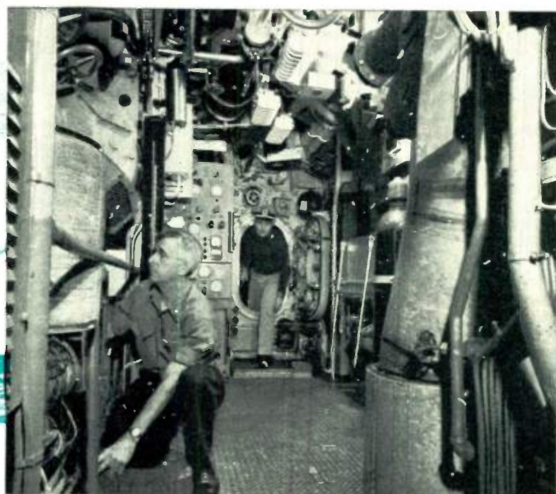
G-E motors and generators, here being readied for sea trials, develop maximum horsepower in minimum space. Lt. Cmdr. F. Andrews, right, will be K-1 captain.
