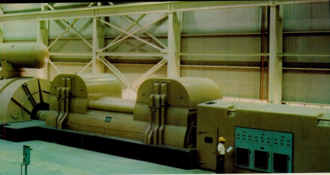
Modern General Electric large steam turbine-generator rated 980,000 KVA installed at Possum Point Station of Virginia Electric Power Company.
