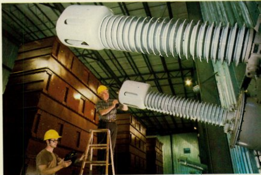
Giant bushings dominate the valve hall of the nation's first solid-state HVDC system in Duluth, Minn., built by GE.
