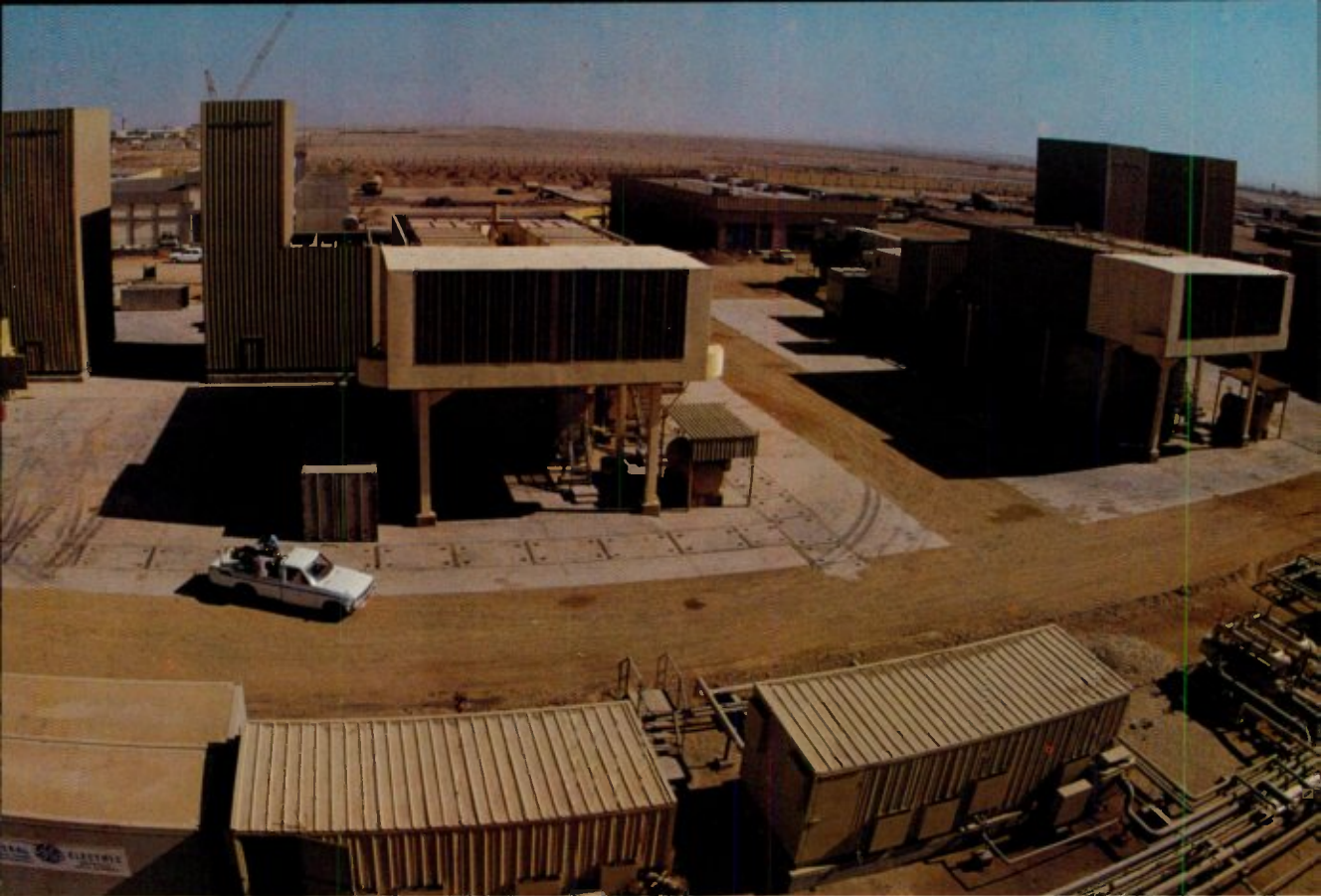
Solution: GE gas turbine complexes such as Jeddah I, shown here, with similar Jeddah II complex underway.
