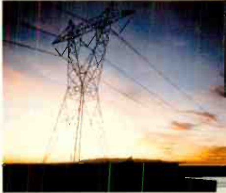
Energy from the Navajo Mine's coal travels via transmission lines throughout the Southwest.
