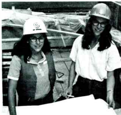
At GE construction site, RECO resident manager Allison Donenfeld, left, and engineering intern Karen Mason pore over blueprints. “People accept you for what you can do,” Donenfeld says, “not what you are.”
