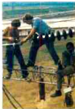
Near Gtaru hydro plant (r) Sadelmi linemen erect transmission tower. Sadelmi supplied the dam's substation and built the towers which bring power to Nairobi.
