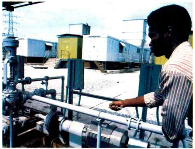
When "brownouts" threatened Lagos last year, emergency electric power was provided by three GE frame-5 gas turbines at Ijora station.
