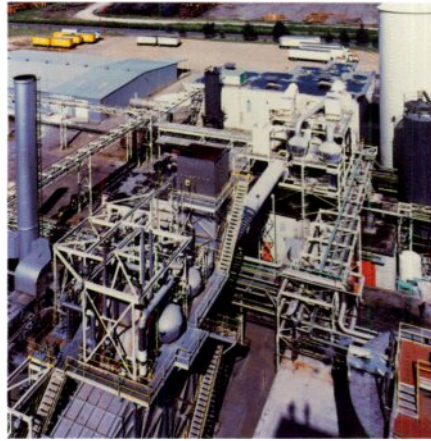
Simpson Paper Company's LM5000-powered cogeneration plant
