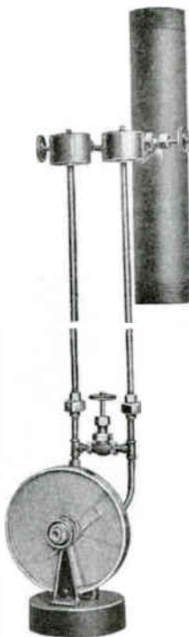
Fig. 4. Indicating Steam Meter and Pipe Connections
