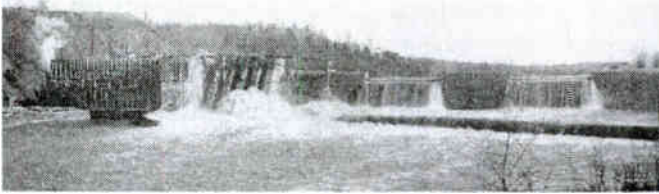
High water during construction, showing water passing over the unfinished sections of the dam spillway
