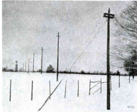
View of the Alternating Current Transmission Pole Line
