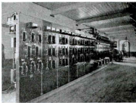
Fig. 4. Switchboard and Exciter in Power House, White Oak Mills
