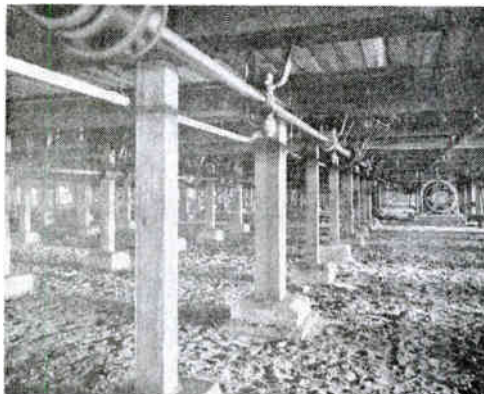
Fig. 5. Ground Floor of Weave Room Showing 150 H.P. Motors Operating Machinery on Floor Above
