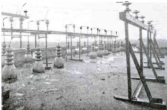
Fig. 10. High Tension Wiring on Roof of Naval Academy Substation
