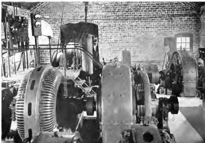
Fig. 19. Coal Hoist Driven by 800-h.p., 350-r.p.m., Direct-current Motor Through Reduction Gears and Controlled by Ward-Leonard System. Synchronous motor-generator set in foreground
