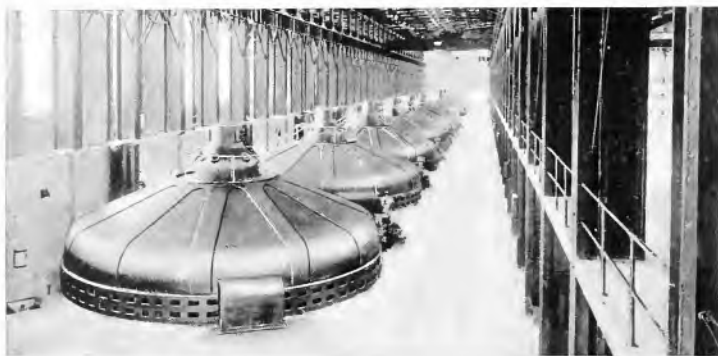
Fig. 5. Nine of the Ten 10,000-kv-a., Three-phase, 6600-volt Cedar Rapids Generators Installed During 1914. Two additional units installed in 1918 are equipped with spring thrust bearings
