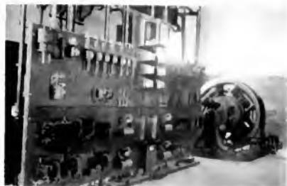
Fig. 10 Automatic Substation Equipment Installed for the Rhode Island Company, Oakland Substation, Controlling Two 300 kw., 600-volt Synchronous Converters
