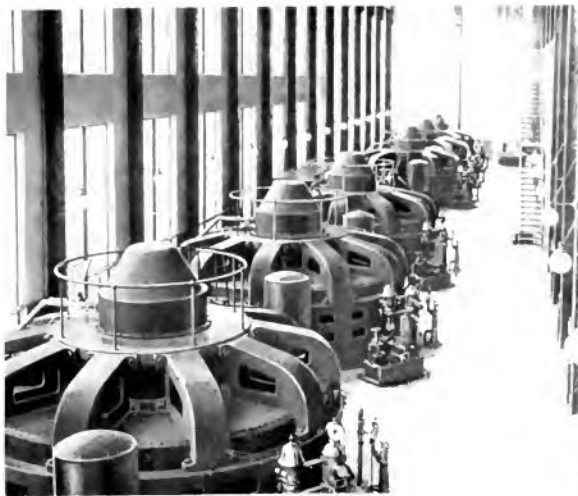
Six 10,000-kv-a., 6600-volt Generators and two 300 kw., 240-volt Exciters at the Volta Plant of the Montana Power Company, Great Falls, Montana. This station supplies power to the Chicago, Milwaukee & St. Paul Railway.
