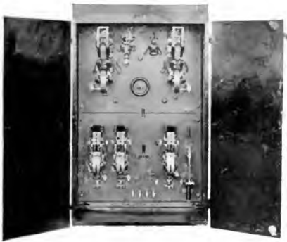
Fig. 9. Starting Panel for Main Circulating Pump Motor
