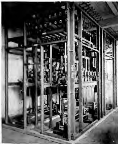
Fig. 4. Combination View of the Port Side and Back of the Control Cell
