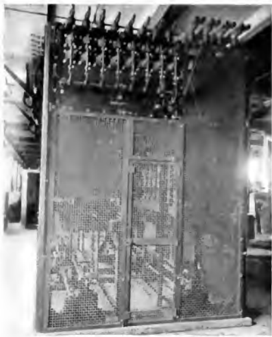
Fig. 5. Starboard Side of the Control Cell, showing protective grille and magnetically locked door
