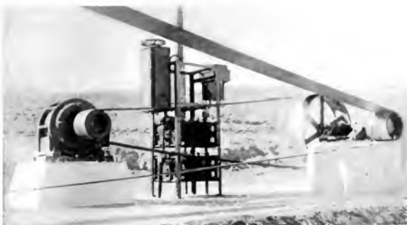
Fig. 3. Another View of the Same Installation Shown in Fig. 2
