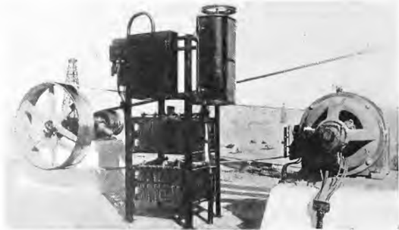
Fig. 2. A Complete 30 15-h.p. Two-speed Oil Well Motor Equipment Installed by a Large Oil Company in Coalinga Field in California. Photograph Made Before Completion of Housing
