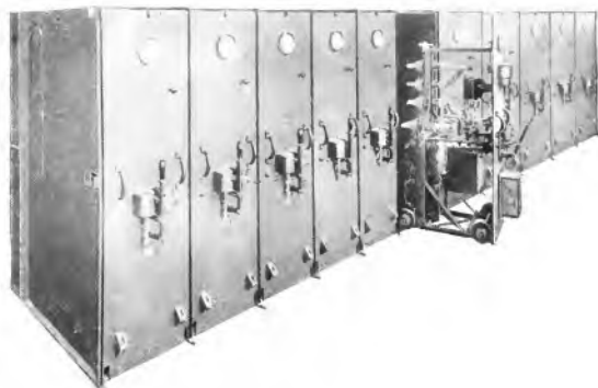
Fig. 24. Removable Truck Safety First Switchboard
