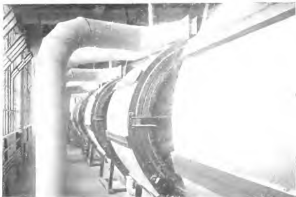
Fig. 2. 600-h.p. Synchronous Motor Operating Dust Collectors
