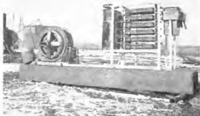
Fig. 8. This Method of Mounting the Entire Electrical Equipment on Skids is Used Extensively for Oil Wells in the Mid Continent Fields
