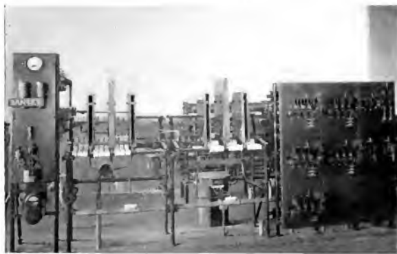
Fig. 9. Installation View of Contactor and Switchboard Panels Used with Induction Motor Driving Mine Hoist, Showing Recent Design of 150-ampere 2200-volt Air-break Primary Reversing Contactors
