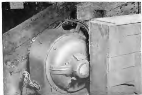
Fig. 6. Mine-type, 25 h.p., 900-r.p.m., 440-volt Squirrel-cage Induction Motor Installed on Crusher at Truesdale, Breaker, D. L. & W. Co.
