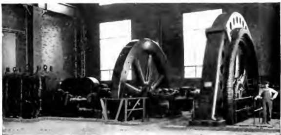
Fig. 6 4000-h.p., 82-r.p.m., 6600-volt, 60 cycle, Single-speed Main-roll Motor Driving 110-in. Plate Mill
