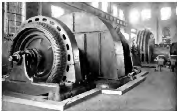
Fig. 17. Motor Room Showing 2500-h.p. Direct-current Reversing Mill Motor and 2000-kw. 2-Unit Flywheel Motor Generator for 36-in. Blooming Mill
