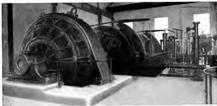
Fig. 13. Double Drum First Motion Hoist Driven by 1800-h.p., 80-r.p.m., D.c. Motor on Tigner-Ward Leonard System Installed at the Elm Orlu Mining Co., Butte, Montana
