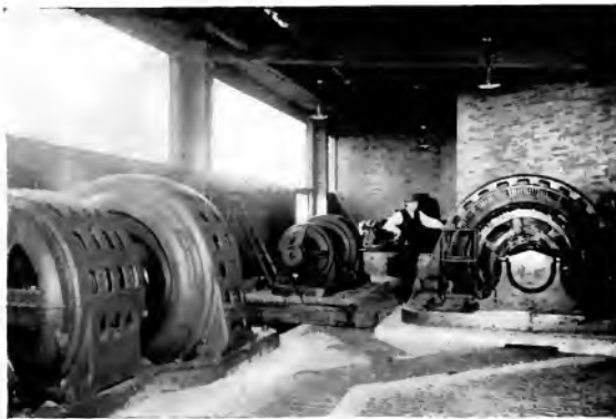
Fig. 14. Motor Room Showing Adjustable Speed Rod Mill Roughing and Finishing Motors with Scherbius Speed Regulating Sets
