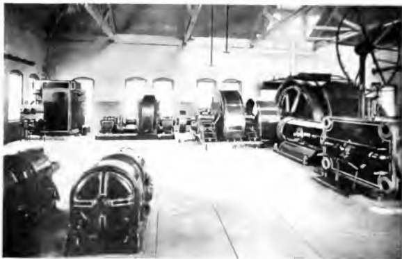
Fig. 6. Largest Induction Motor Driven Hoist in America. 1800 h.p., 360 r.p.m., 2200-volt Motor Gearing to 12-ft. Diameter Hoist Drum, Controlled by Liquid Rheostat Shown in Left Back-Ground. Hoist Originally Driven by First Motion Corlist Steam Engine. Tennessee Coal, Iron & R. R. Co., Muscoda, Ala.
