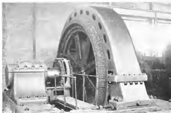
Fig. 3. 3500-h.p., 92-r.p.m., 2200-volt, 60 cycle, Single-speed Main-roll Motor Driving a Continuous Mill
