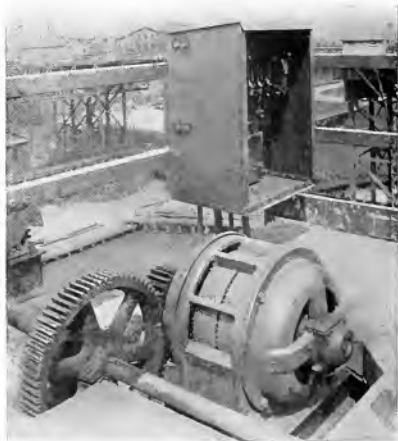
Fig. 20. Control Panel and Motor Geared to Line Shaft Which Operates Twelve Small Hoists for Lifting Spouts, Duluth & Iron Range R. R. Docks, Two Harbors, Minn.
