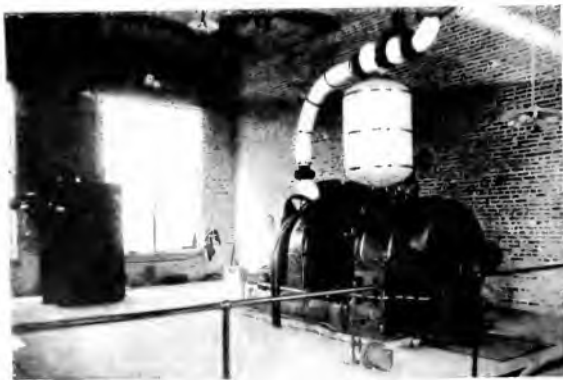
Fig. 8. 375 kw. Curtis Steam Turbine Installed at C. Reiss Coal Company's Dock in Manitowoc, Wis.
