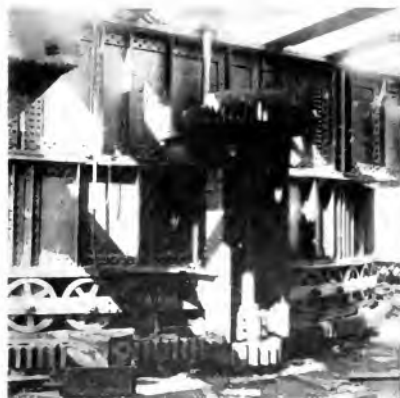
Fig. 1. Driving Mechanism on a Swing Span Bridge Note small wheels on which weight of span is carried.
