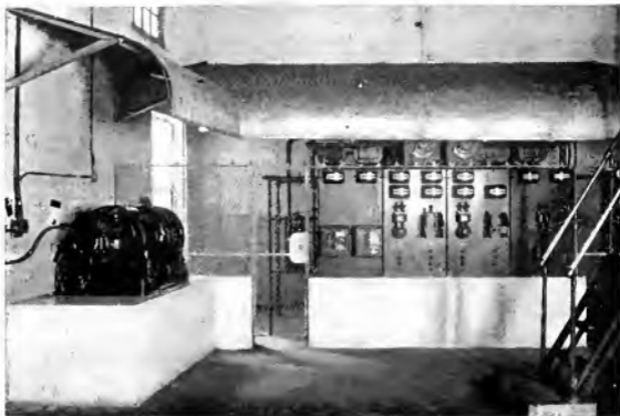
Fig. 3. Control Board and Motor-generator Exciter Set for Machines in Fig. 5
