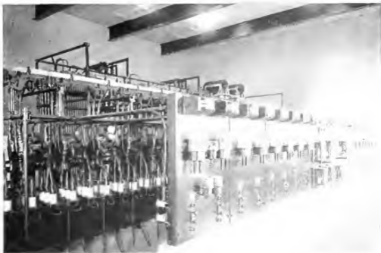
Fig. 1. Front View of Switchboard in New Main Substation, Cudahy Packing Co., Omaha, Neb.
