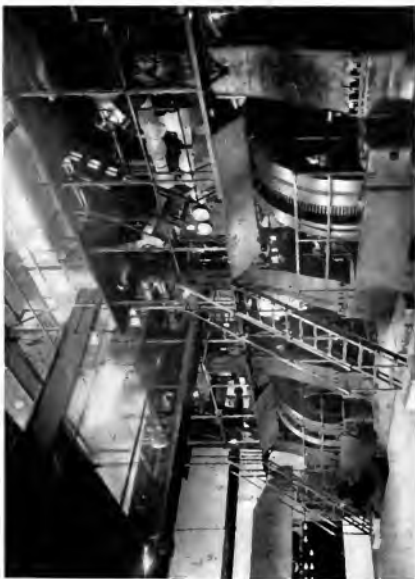
Fig. 5. Two 300-ton Refrigerating Machines Driven by Two 500-k.v.a. each, 6600-volt, 3-phase, 60 cycle General Electric Synchronous Motors
