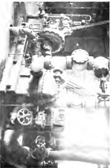
Fig. 12. Turbine Power Converter of a Hydro-Pump.
