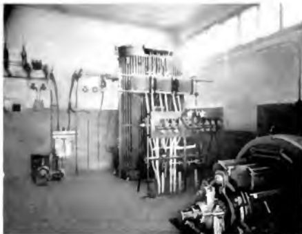
Fig. 7. Transformers, Converter and Auxiliaries
