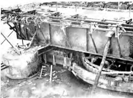
Fig. 8. Lowering House and Pouring Concrete at the Same Time Level of fresh concrete was kept about one foot out of water
