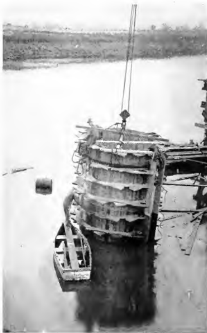
Fig. 4. Landing Form for One of the Four Supporting Piers. These forms were 10 ft. dia. and 26 ft. long
