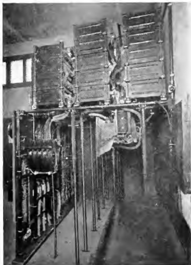
Fig. 4. Back of Switchboard, with Resistors Above, Heavy Contactors in Center, and Controller Cover in Foreground
