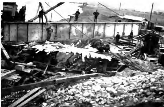
Fig. 5 One of the Four Girders from which the House was Lowered: 7 ft. deep, 67 ft. long, weight 14 tons.
