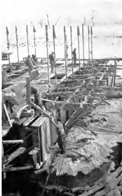
Fig. 7. Operating the Ratchet Lowering Wrenches by Lines Led to the Two Derricks
