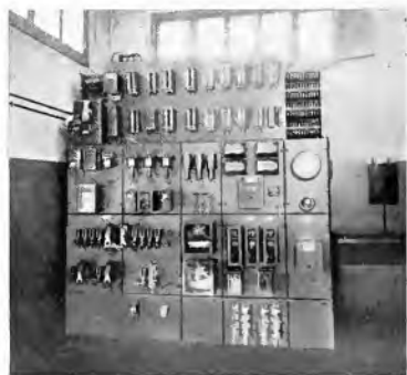
Fig. 5. Main Switchboard with Controller in Background
