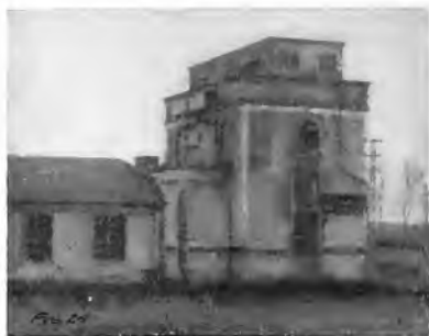
Fig. 24. 2000-kw., 65,000 11,000 volts, Three-phase, 50-cycle Substation of the Compagnie Lorraine d'Electricite Between Void and Commercy, in operation throughout the war. It supplied several large American units with electric current. The main 65,000-volt line passing through this station fed the extensive army lines in the Verdun sector from a similar substation at Bar-le-Duc.
