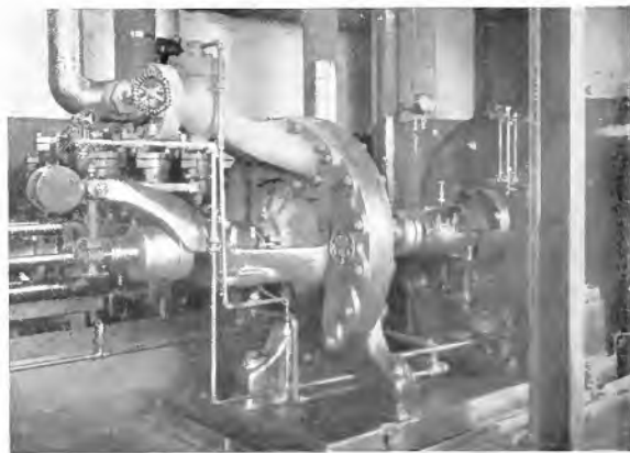
Fig. 1. Short-arc Single-stage Turbine Driving Centrifugal Air Pump on Condenser
