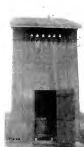
Fig. 26. French Army Transformer Station. Of the same type as shown in Fig. 25, but with the door open showing transformer sitting on masonry foundation and insulated stool for operator to stand on. 6000-volt, three-phase incoming line shown on pole behind the house. Aviation field barracks in rear.
