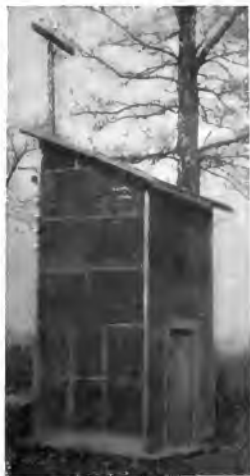
Fig. 25. French Army Transformer Station. Wooden building which can be moved complete with switches, insulators, choke coils, lightning arresters, etc., on auto truck without dismantling. A great many were used in all the French and American Army areas. 6000-volt line shown above and regular 190 110-volt, four-wire distributing lines below.
