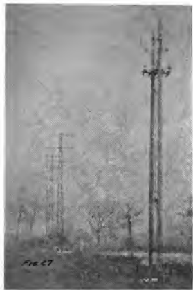
Fig. 27. Abandoned High Voltage Line Steel Poles Used for Military Line to Aviation Field. Branch line taken off with French three-pole air-brake switch mounted between the tops of two wooden poles with operating lever down alongside one of them. This Army line was for 6000 volts, three-phase, with three transformer stations
