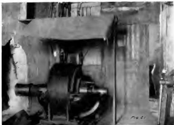
Fig. 21. St. Mihiel Electric Plant. The generator in the building shown in Figs. 19 and 20. Note wooden frame switchboard behind the generator and the hood over it to deflect dripping rain.
