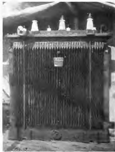
Fig. 13. Captured Boche Three-phase Transformer. Rating plate missing. Thought to be about 50 kv. a., 17000 3000 volts
