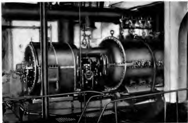
Fig. 4. Photograph of the Turbo Compressor as Installed
