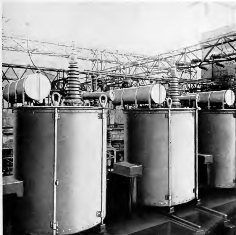
OUTDOOR INSTALLATION OF TRANSFORMERS FITTED WITH OIL CONSERVATORS
