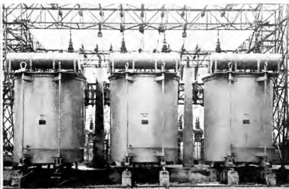
Fig. 8. View of Transformer Bank No. 1 at the Canton Station of the American Gas and Electric Co.
