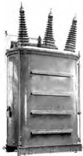
Fig. 2. High-voltage Side of a Larger High-voltage Three-phase Transformer Provided with Oil Conservator
