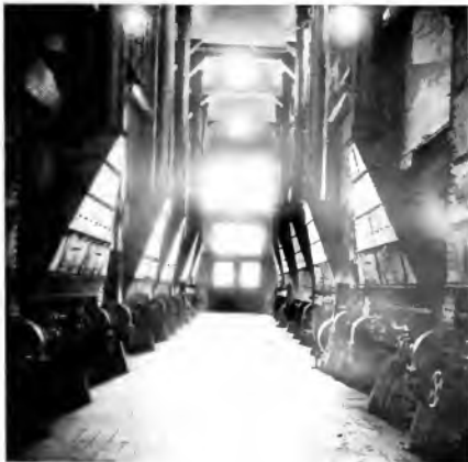
Fig. 7. State St. Station; United Electric Light Co., Boiler Room
