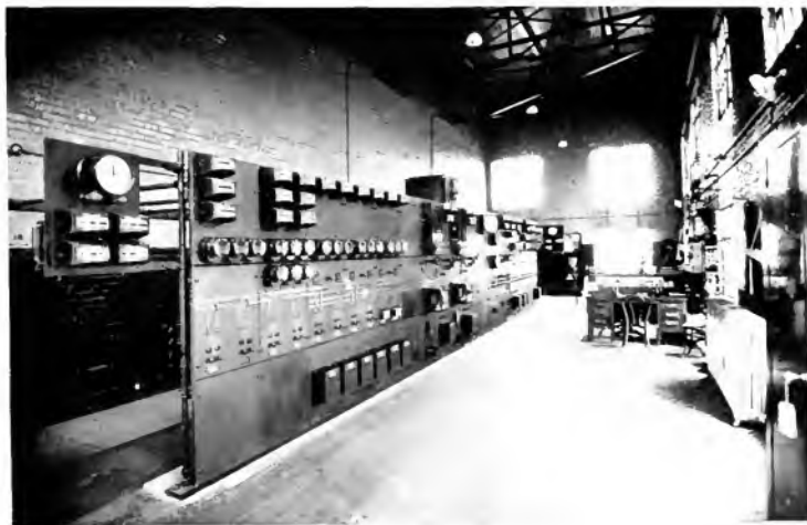
Fig. 2. View of Switchboard at the Warrior Steam Plant
