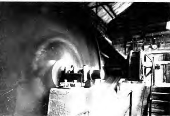
Fig. 7. The turbine shaft comes through a stuffing box in the wall. This induction generator has pumped 126,800 kw-hr. into the power system of the steel plant
