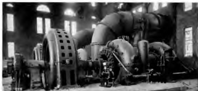
Fig. 1 Interior View of the Long Lake Station of the Washington Water Power Company, near Spokane, Washington, showing two 22,500-h. p. turbines designed for a head of 168 ft. at a speed of 200 r. p. m. A third unit is now being installed
