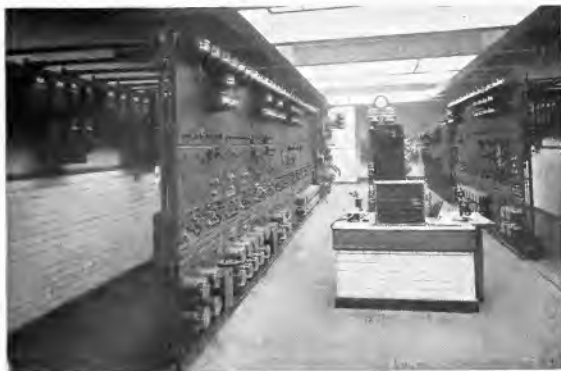
Fig. 10. State St. Station, United Electric Light Co. Switchboard Room
