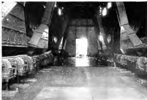
Fig. 14. Firing Aisle, Boiler Room; Hampden Station
