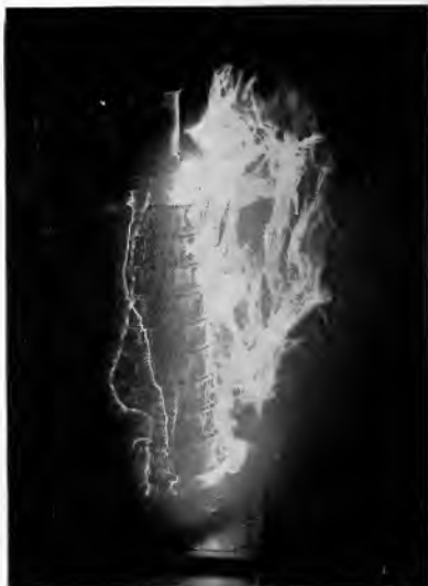
Fig. 7. Wet Flashover of F3 Bushing at 305,000 Volts
