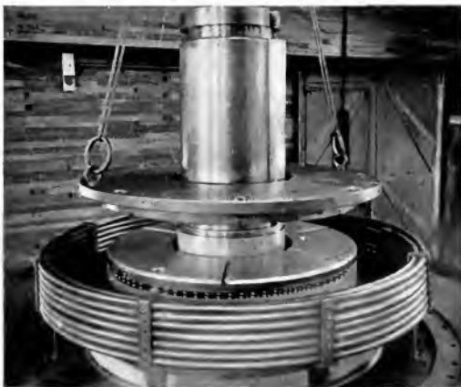
Fig. 3. Spring Thrust Bearing and Cooling Coils to Support Load of 550,000 Lbs., Cedars Rapids Power Station
