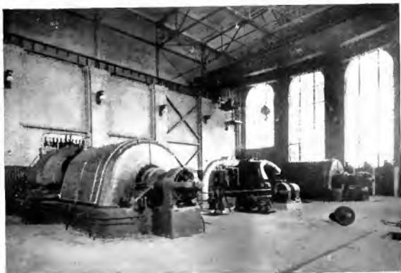
Fig. 15. Turbine Room, 15,000 kw. Units; Hampden Station
