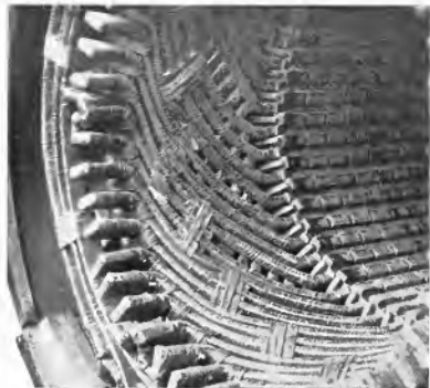
Fig. 2. An Early Type of Turbine Alternator Armature with Insufficient Bracing of the End Windings, showing effects of short circuit at normal voltage. Note grouping of coils by phases
